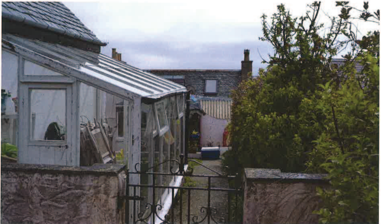
Figure 25 : Corrugated Materials on Extension (argyll terrace)
