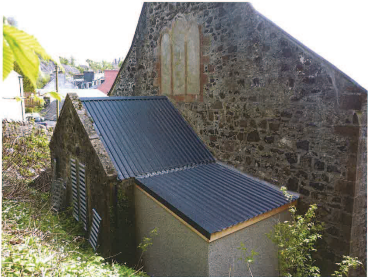
Figure 4 : Profiled Metal sheet roof on Listed Building (the Gallery) on Main Street
